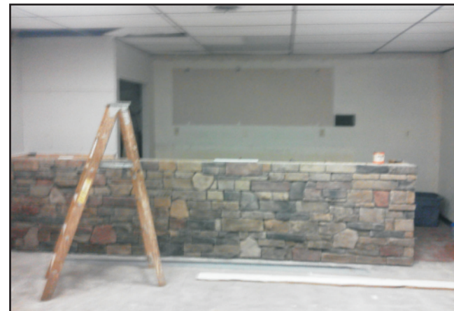
Construction of the upper rooms began immediately after the tripe dinner. Above - The bar in the upper room gets a face lift and storage room.
